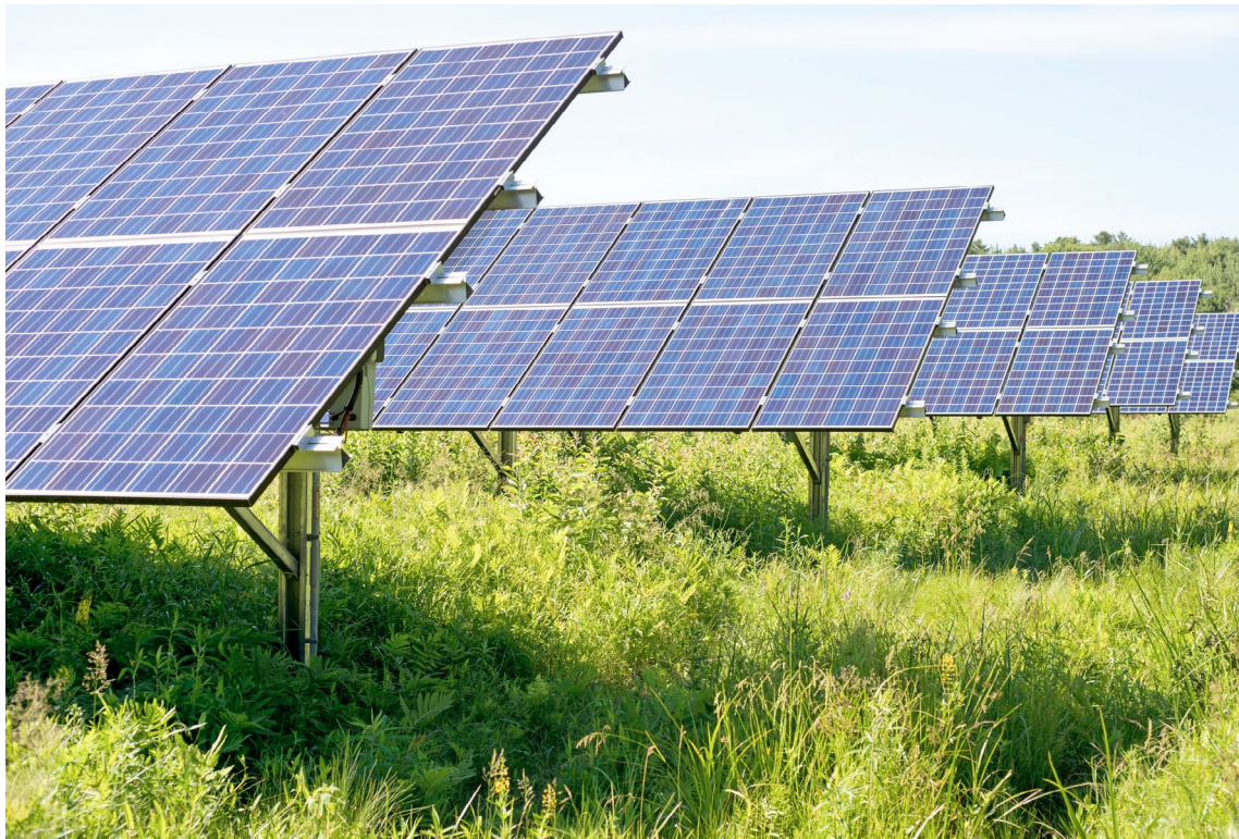
A solar photovoltaic farm generating electricity. The City needs to make investments in solar projects for it to achieve its goals. Photo: U.S. Department of Energy
