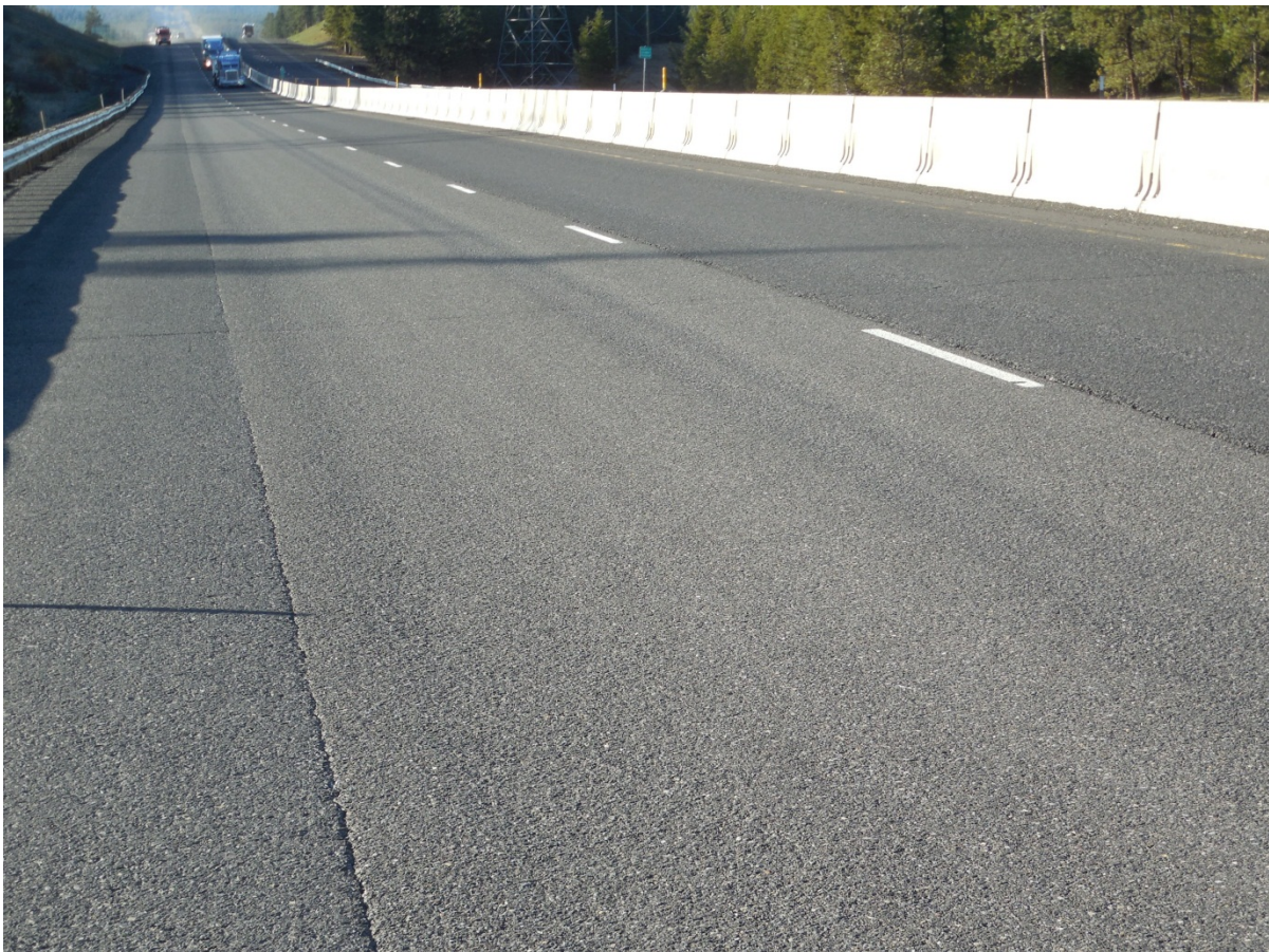
Figure 4.1: I-84 West of La Grande: The dual rut caused by heavy load trucks can be seen.
