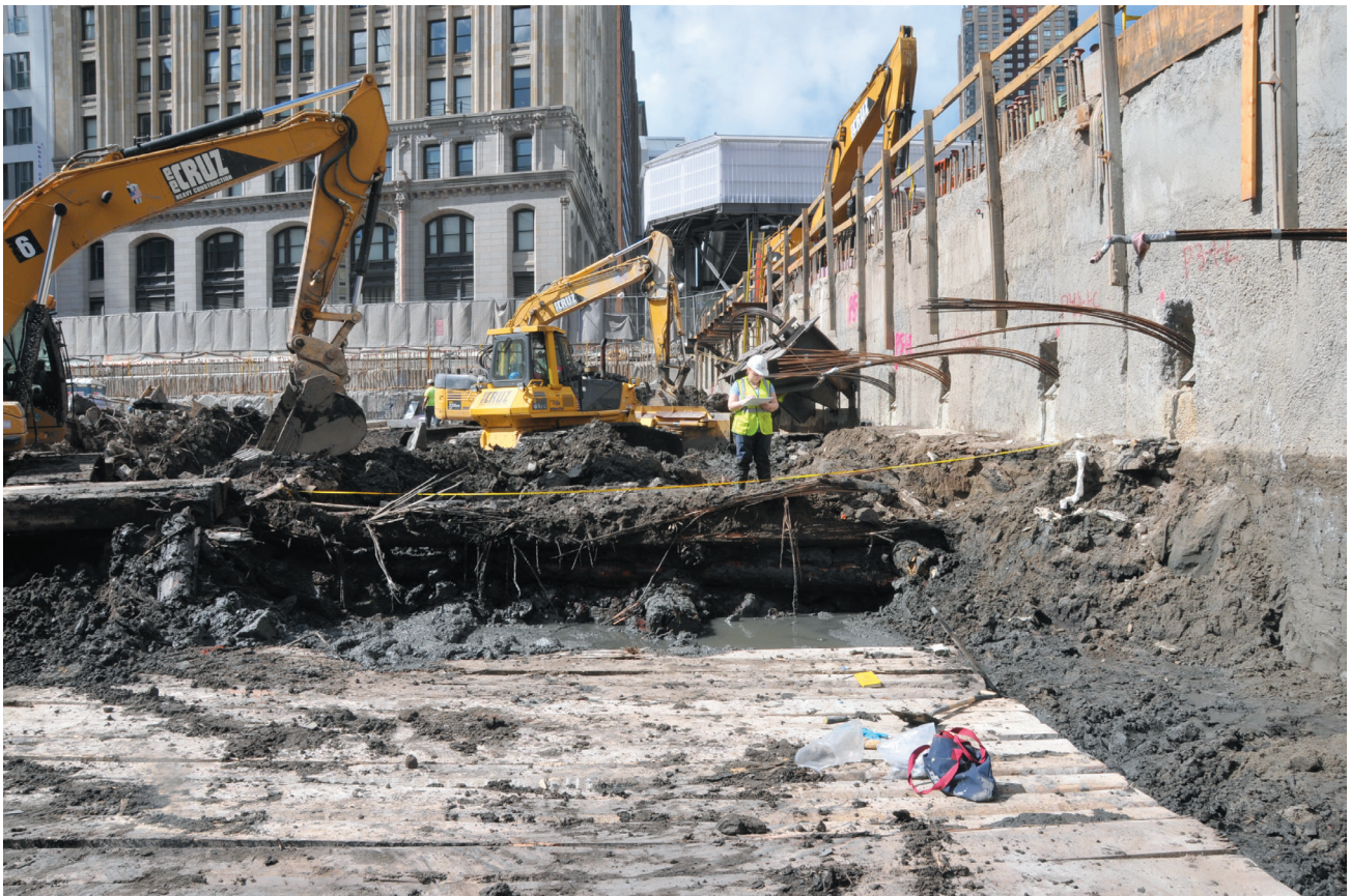
Photograph of 2010 monitoring during excavation of the World Trade Center Vehicular Security Center Project. Photograph by AKRF, courtesy of LMDC.
