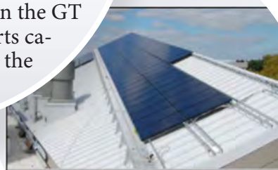
Rockville Campus Science Center Photovoltaic Array
