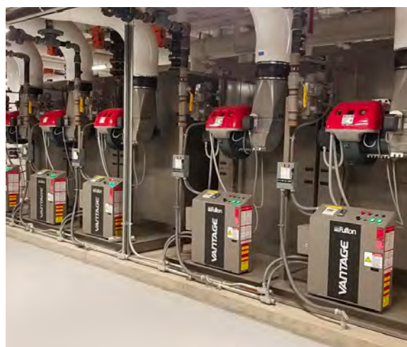
High Performance Hot Water Heating Plant Long Nguyen Kimmy Doung Student Services Building Rockville Campus
