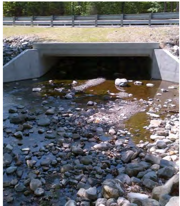
This stream crossing on Bottle Brook in Kingsbury Plantation is an example of a climate-ready infrastructure project that is also geared to improve habitat connectivity.
