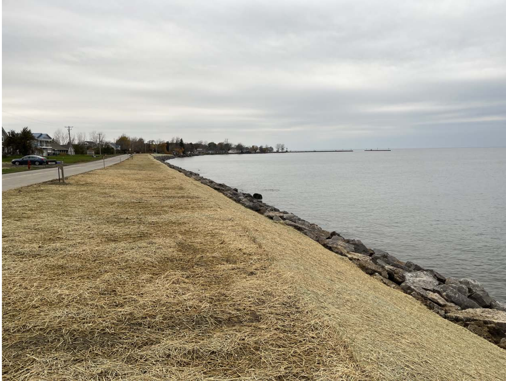
Pictured above, the completed Lakeside Road West flood resiliency project, which included the construction of a new access road and the installation of rip rap stone to stabilize the shoreline and protect the public water line, is seen.
