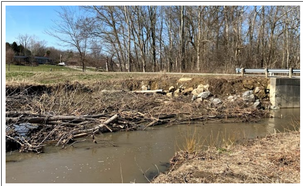
Note evidence of failed rock protection project. Photo Source: Ben Sperry, OU, March 2021
