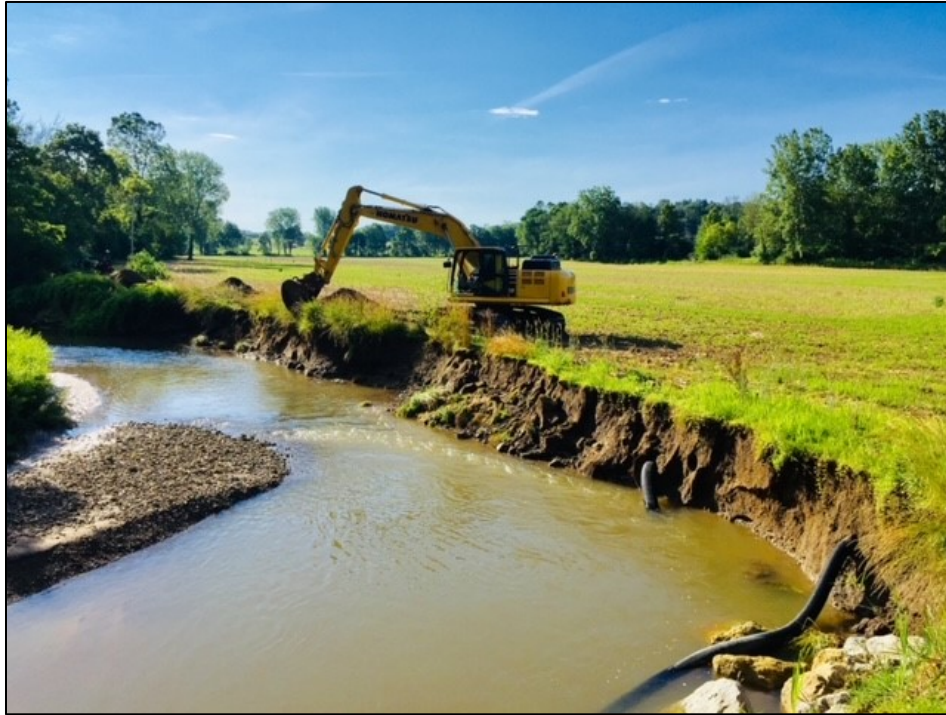
[a] View during early stages of construction facing upstream from bridge. Note significant erosion of channel on right side of view. Photo Source: Ron Wine, CMS, June 2019
