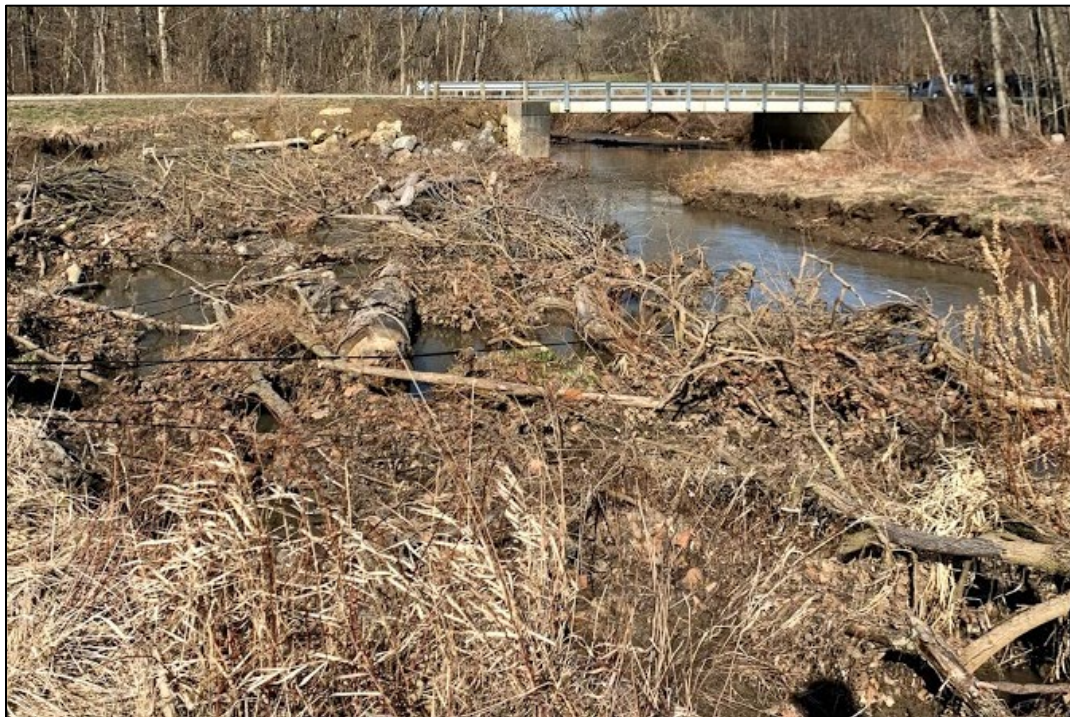
[b] Post-Construction view looking downstream towards bridge structure with Palmiter installation completed. Photo Source: Ben Sperry, OU, March 2021
