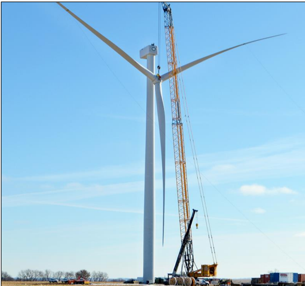
Image 1: Cuming County Public Power District purchases electricity from this 2.5 MW GE wind turbine with an 89-meter hub height and a 127-meter rotor diameter. Photo credit: Boyd Jones
