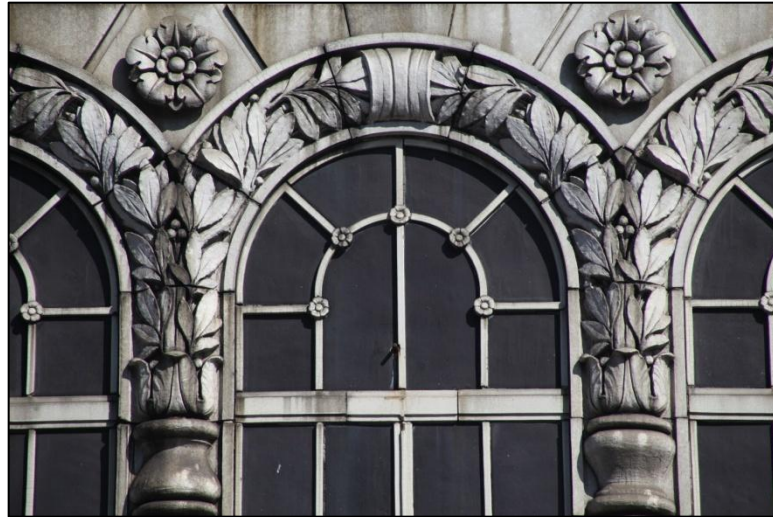
Loew's Canal Street Theatre Details of terra-cotta ornament Photo: Christopher D. Brazee (2009)
