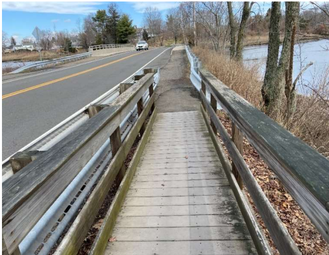
Exhibit 26: Gap between the boardwalk and the sidewalk along the bridge
