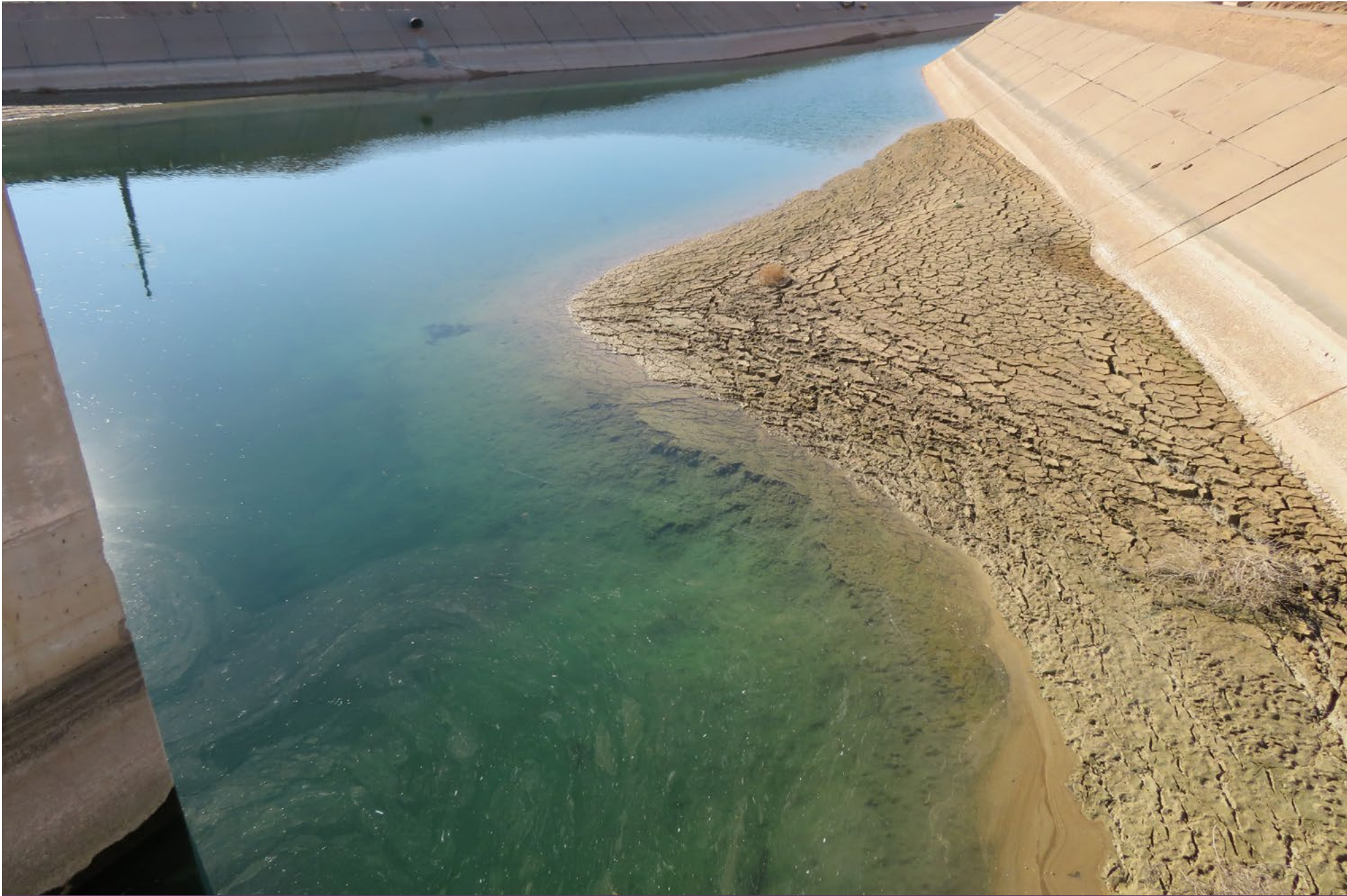
SEDIMENT DEPOSITION AT BRD; SHOWN HERE WITH LOW WATER LEVELS.
