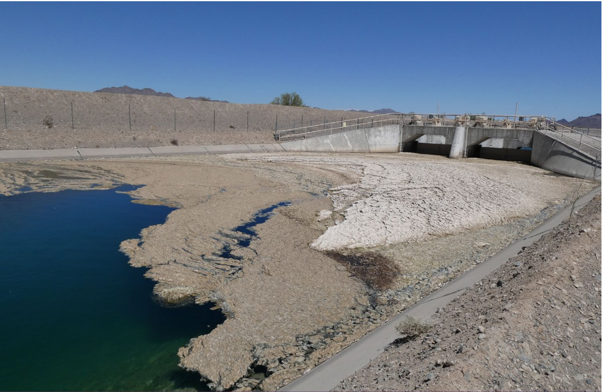
CYMBELLA ACCUMULATED UPSTREAM OF CHECK #3 WHEN FLOWS WERE CURTAILED IN JULY 2022. THIS MAY HAVE PREVENTED PROBLEMS WITH CLOGGED STRAINERS DOWNSTREAM AT LHQ.
