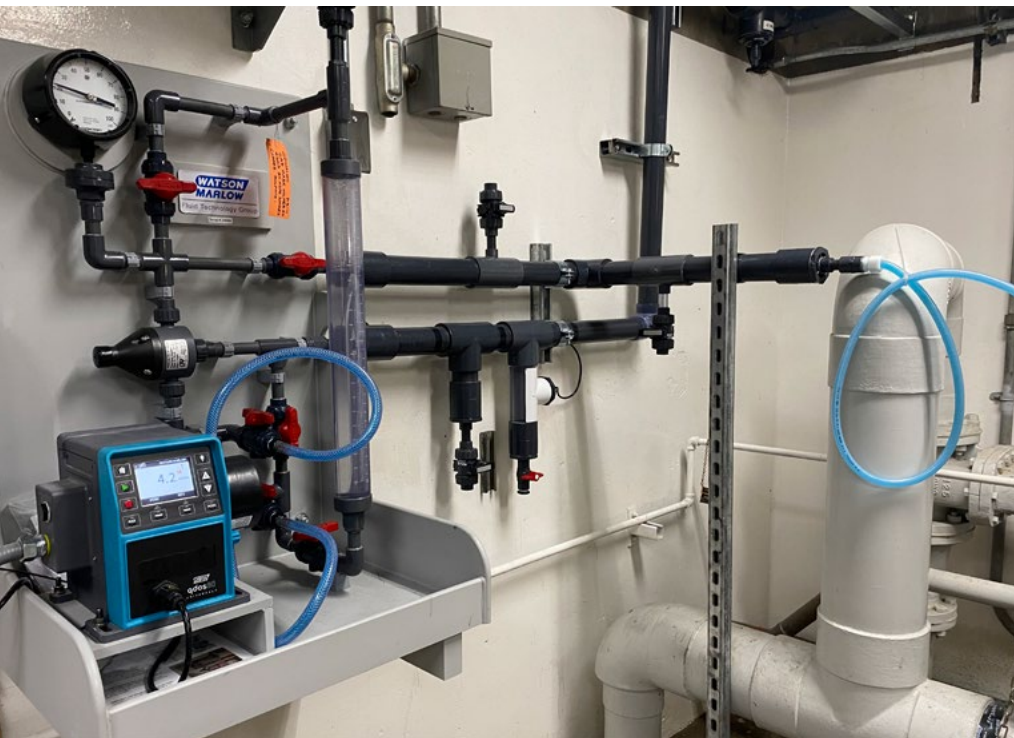
CHEMICAL INJECTION SYSTEM AT MWP
