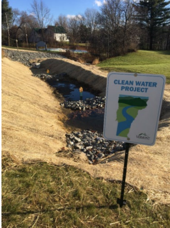
Hazen Union School stormwater gravel wetland funded by DEC's Clean Water Initiative Program
