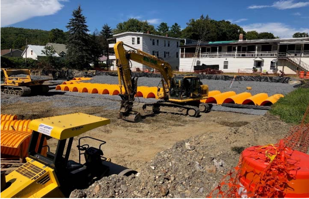
Figure 28. Installation of sub-surface infiltration chambers treats runoff along Water Street in the Town of Northfield. Project funded by a DEC Clean Water Initiative Program grant. (Source: Central Vermont Regional Planning Commission)
