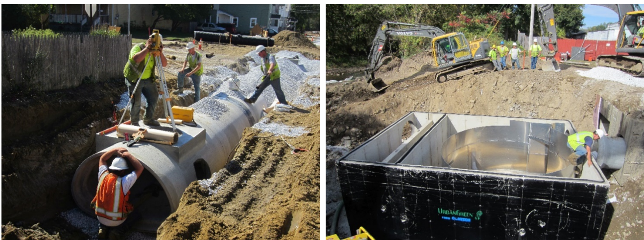
Figure 32. Installation of a reinforced concrete pipe (left) and stormwater separation system (right) to abate combined sewer overflows (CSOs) in the City of Rutland. Project financed by the Clean Water State Revolving Fund. (Source: Otter Creek Engineering)
