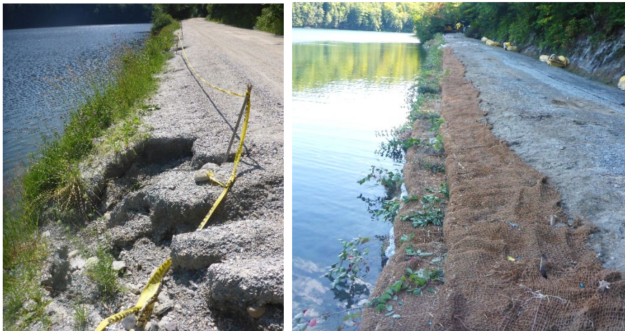
Figure 34. Before (left) and after (right) the installation of encapsulated soil lifts to naturally stabilize and reduce erosion along Black Pond Road in Town of Hubbardton. Project funded by a DEC Clean Water Initiative Program grant. (Source: Northwoods Stewardship Center)
