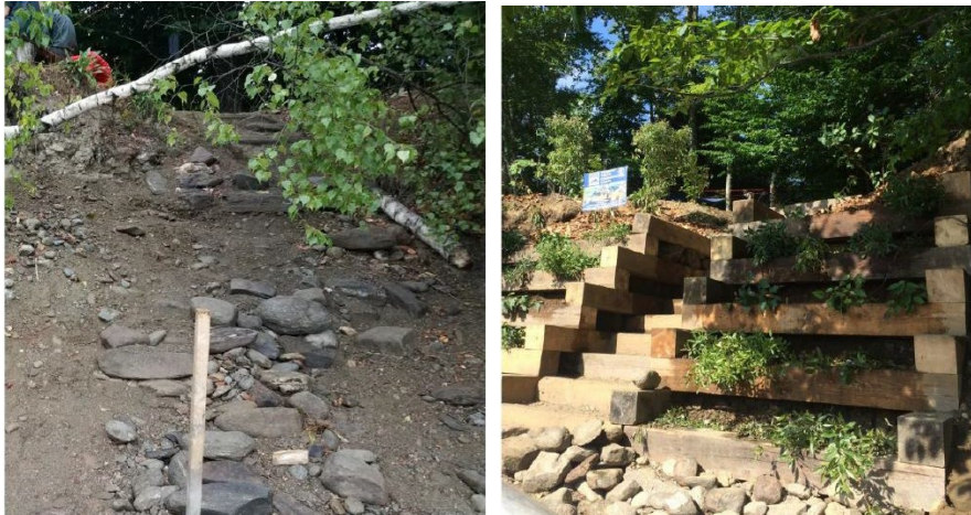
Figure 36. Before (left) and after (right) the installation of Vermont's first crib-wall staircase to remediate erosion at a lakeshore access point in Waterbury Center State Park. Project funded by DEC Clean Water Initiative Program grant. (Source: Vermont Youth Conservation Corps)
