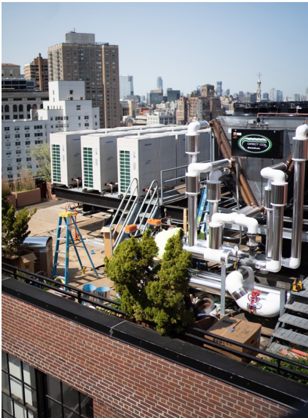
Air-to-water heat pumps on roof of 111 4th Avenue
