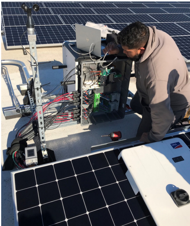
A contractor commissions the solar panels at NYPL’s Charleston Branch Library in Staten Island, the first library in New York City designed for net-zero energy. Source: DCAS
