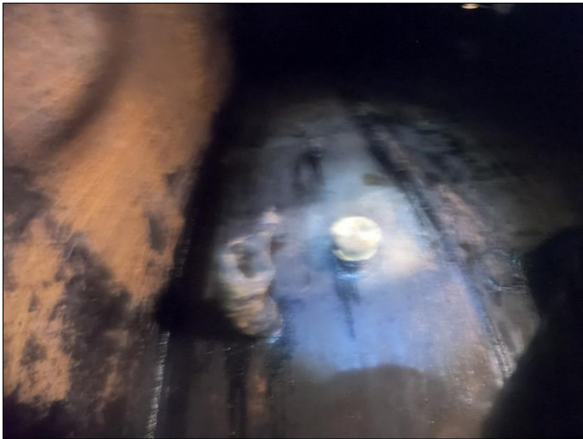
Figure 22. Penetrations sealed at the outboard bulkhead in A-26F.
