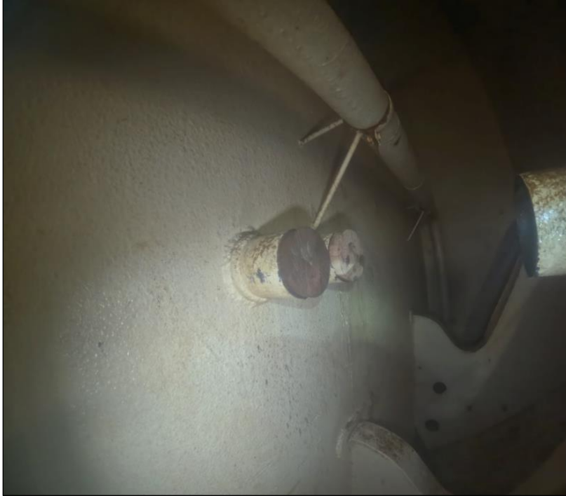
Figure 31. A 3.5" ballast and a 4.0" fuel pipe penetrations sealed at the inboard bulkhead in A-33F at FR 52-53.
