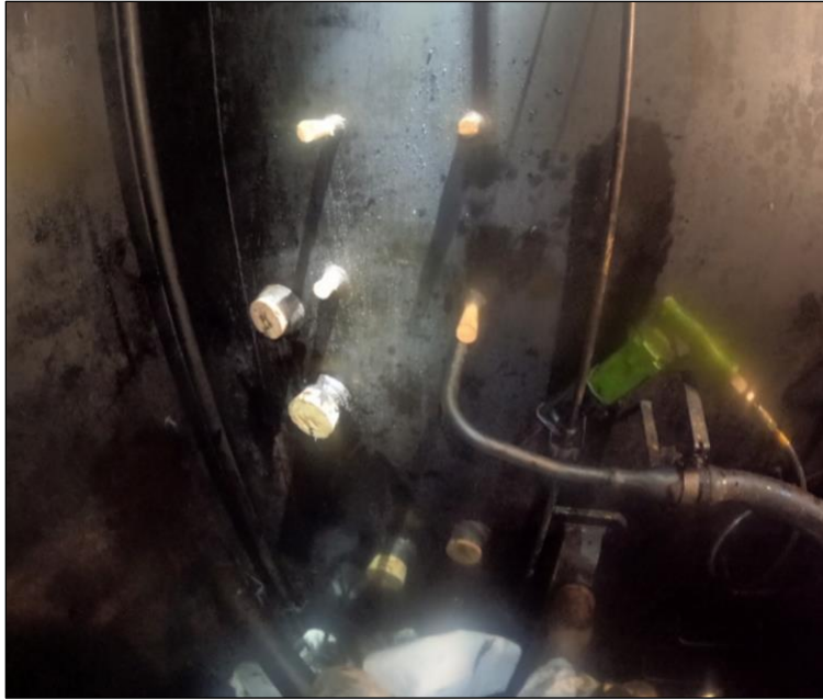
Figure 17. Penetrations sealed at the inboard bulkhead in A-21F.
