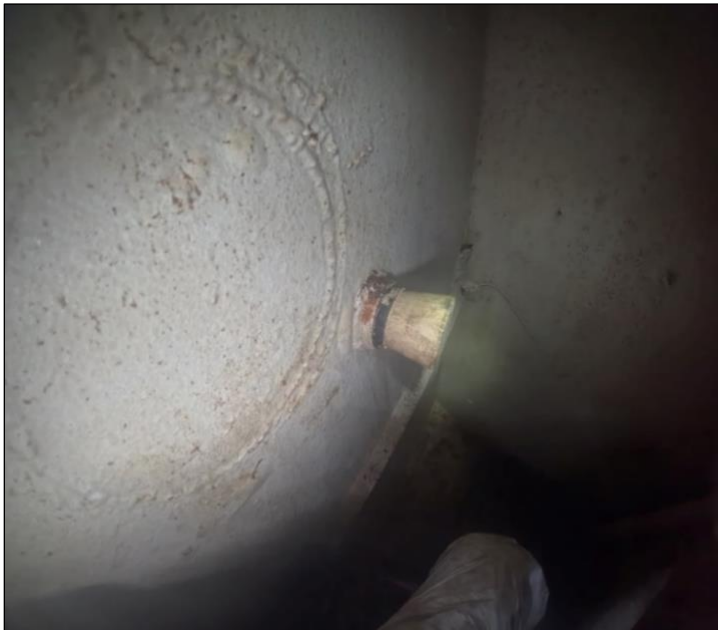
Figure 29. A 2.5" penetration sealed at the outboard bulkhead in A-33F at FR 55-56.
