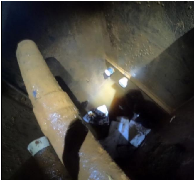
Figure 35. Ballast pipe and fuel oil pipe penetrations to A-46.5F sealed at the outboard bulkhead in A-44V. Photograph captured in A-44V.
