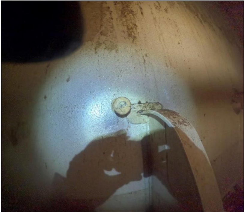
Figure 28. A 3.5" ballast pipe penetration sealed at the outboard bulkhead in A-32F at FR 52-53.
