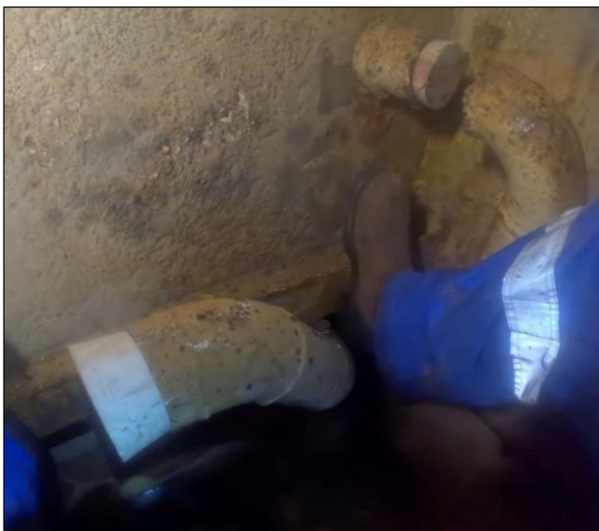
Figure 40. Ballast pipe and fuel oil pipe penetrations sealed at the inboard bulkhead in A-54F. Photograph captured in A-54F.
