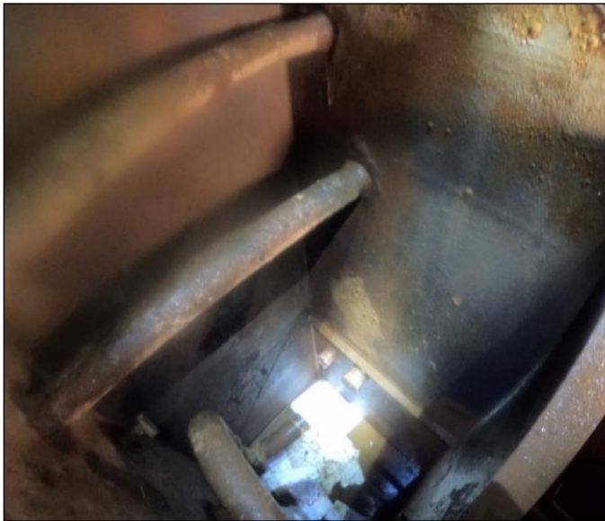
Figure 39. Ballast pipe and fuel oil pipe penetrations to A-54.5F sealed at the outboard bulkhead in A-52V. Photograph captured in A-52V.
