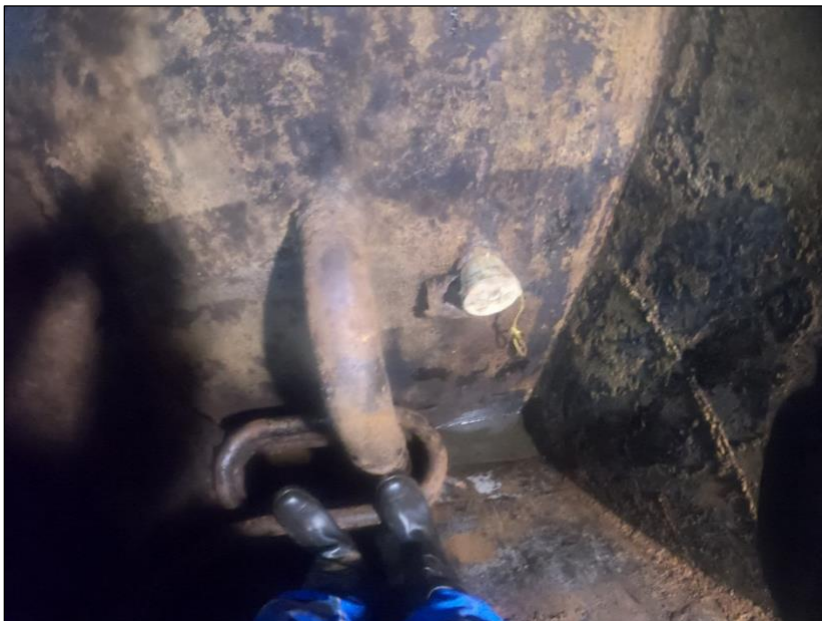
Figure 20. Sealed ballast line at the inboard bulkhead in A-26.5F – photograph captured in A-26.5F.
