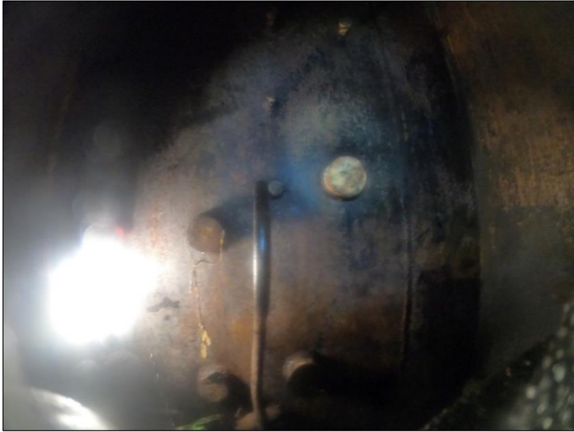
Figure 21. Penetrations sealed at the inboard bulkhead in A-26F.
