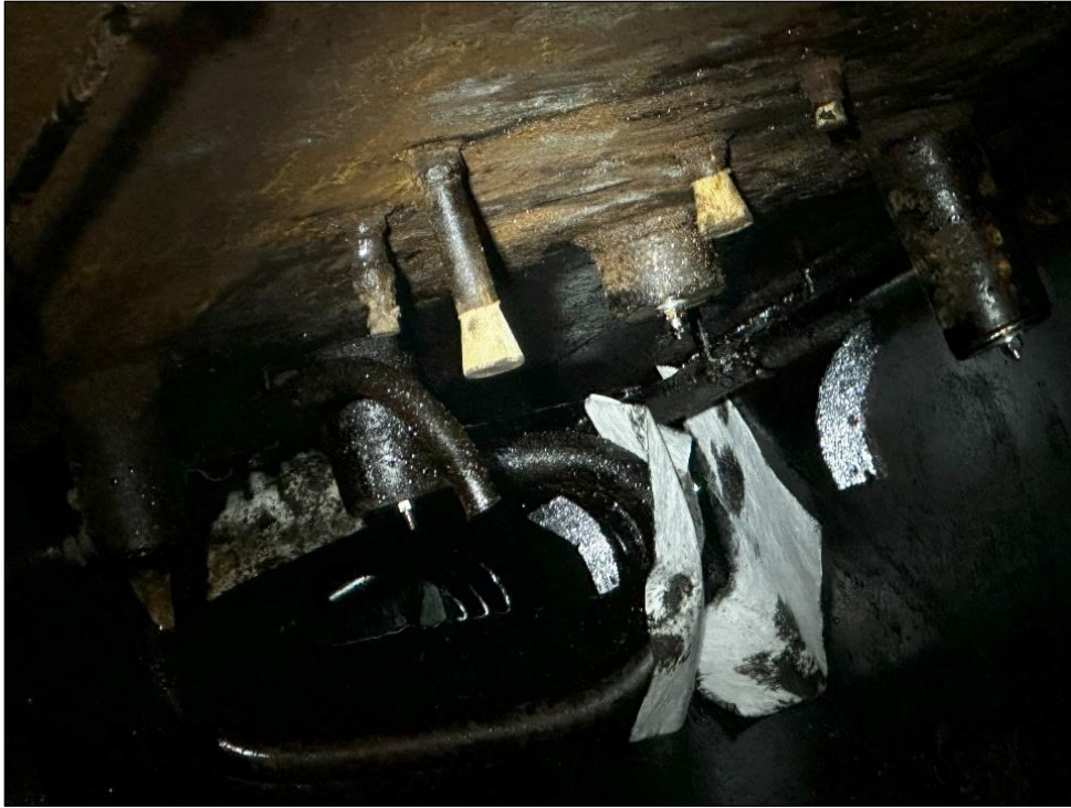
Figure 15. Penetrations sealed at the inboard bulkhead in A-20F.
