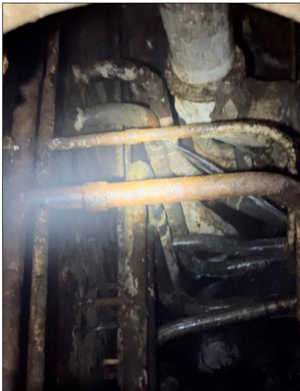
Figure 1. Leaking piping in tank A-28V.
