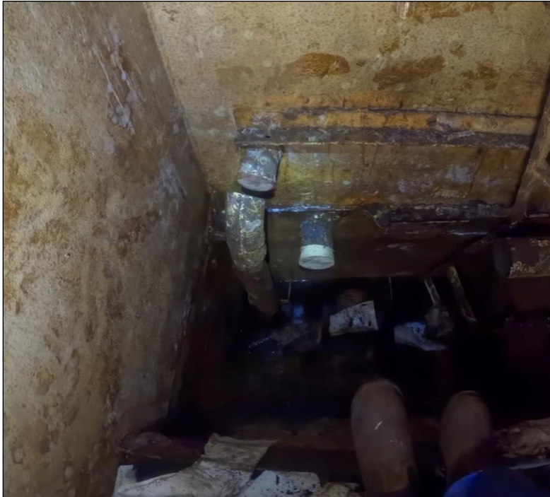
Figure 41. Ballast pipe and fuel oil pipe penetrations sealed at the inboard bulkhead in A-55F. Photograph captured in A-55F.
