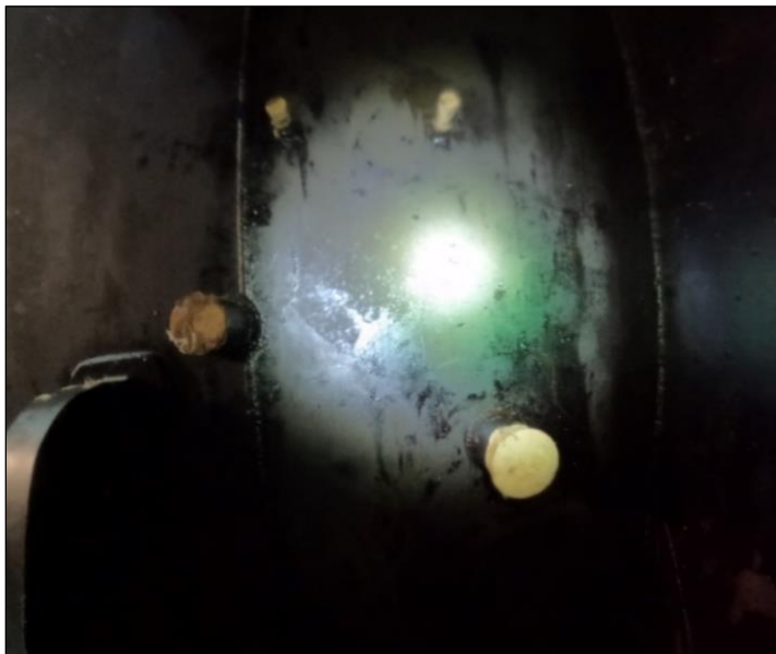
Figure 24. Penetrations sealed at the outboard bulkhead in A-21F.
