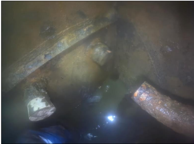
Figure 37. Ballast pipe and fuel oil pipe penetrations to A-47.5F sealed at the outboard bulkhead in A-45V. Photograph captured in A-45V.
