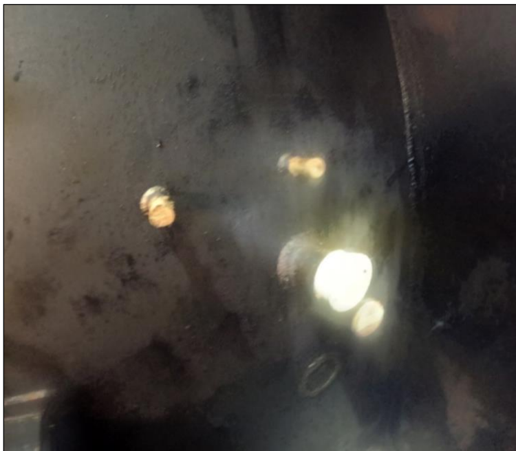
Figure 18. Penetrations sealed at the outboard bulkhead in A-21F.
