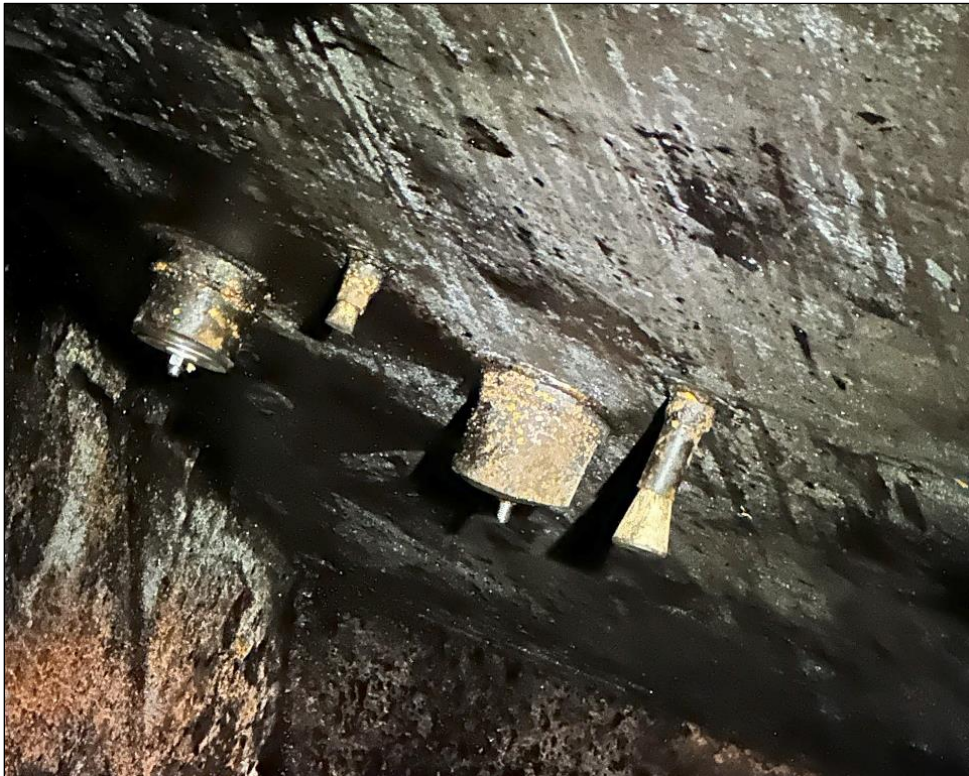
Figure 16. Penetrations sealed at the outboard bulkhead in A-20F.
