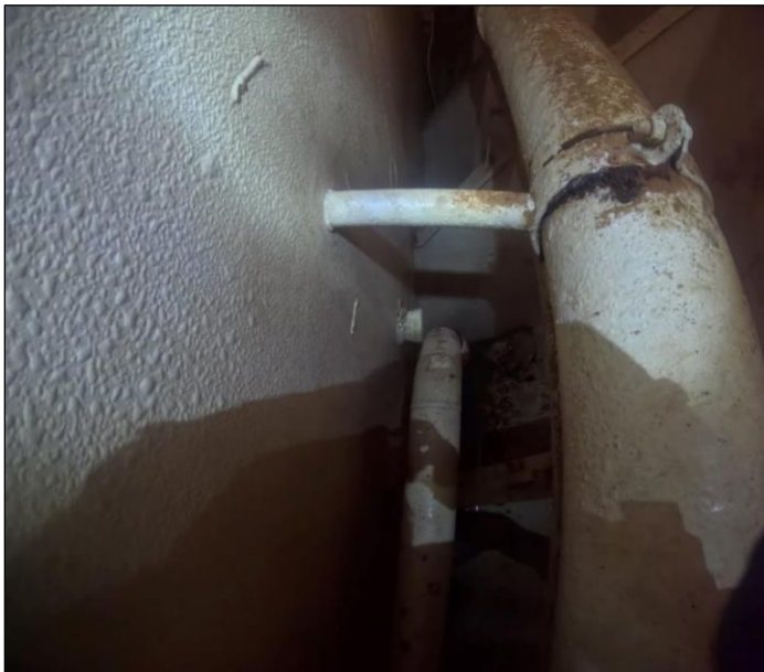
Figure 26. A 3.5" ballast pipe penetration sealed at the inboard bulkhead in A-32F at FR 55-56.
