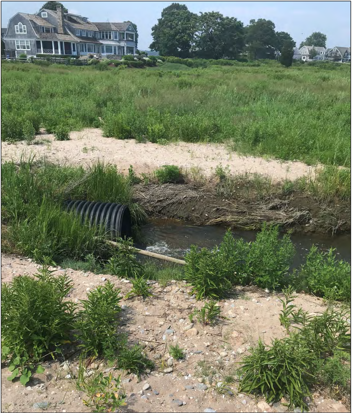
Figure 15 2019 Winter Storm Emergency Response Project: Corrugated pipe (eastern end of the pipe) during ebb flow conditions
