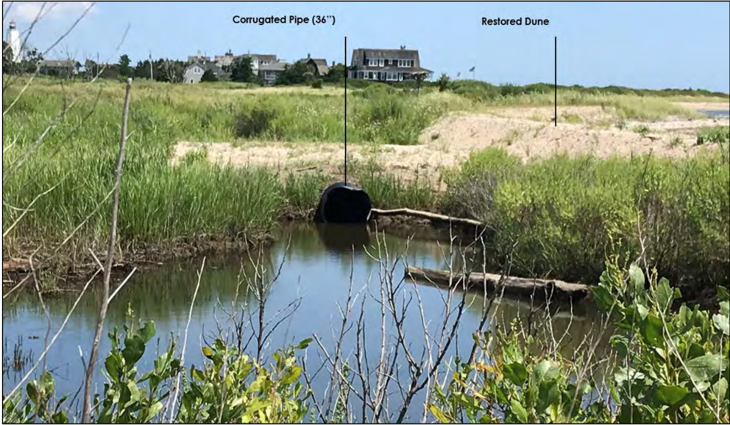
Figure 14 2019 Winter Storm Emergency Response Project: Corrugated pipe (western end of the pipe) to restore tidal connectivity and dune restoration
