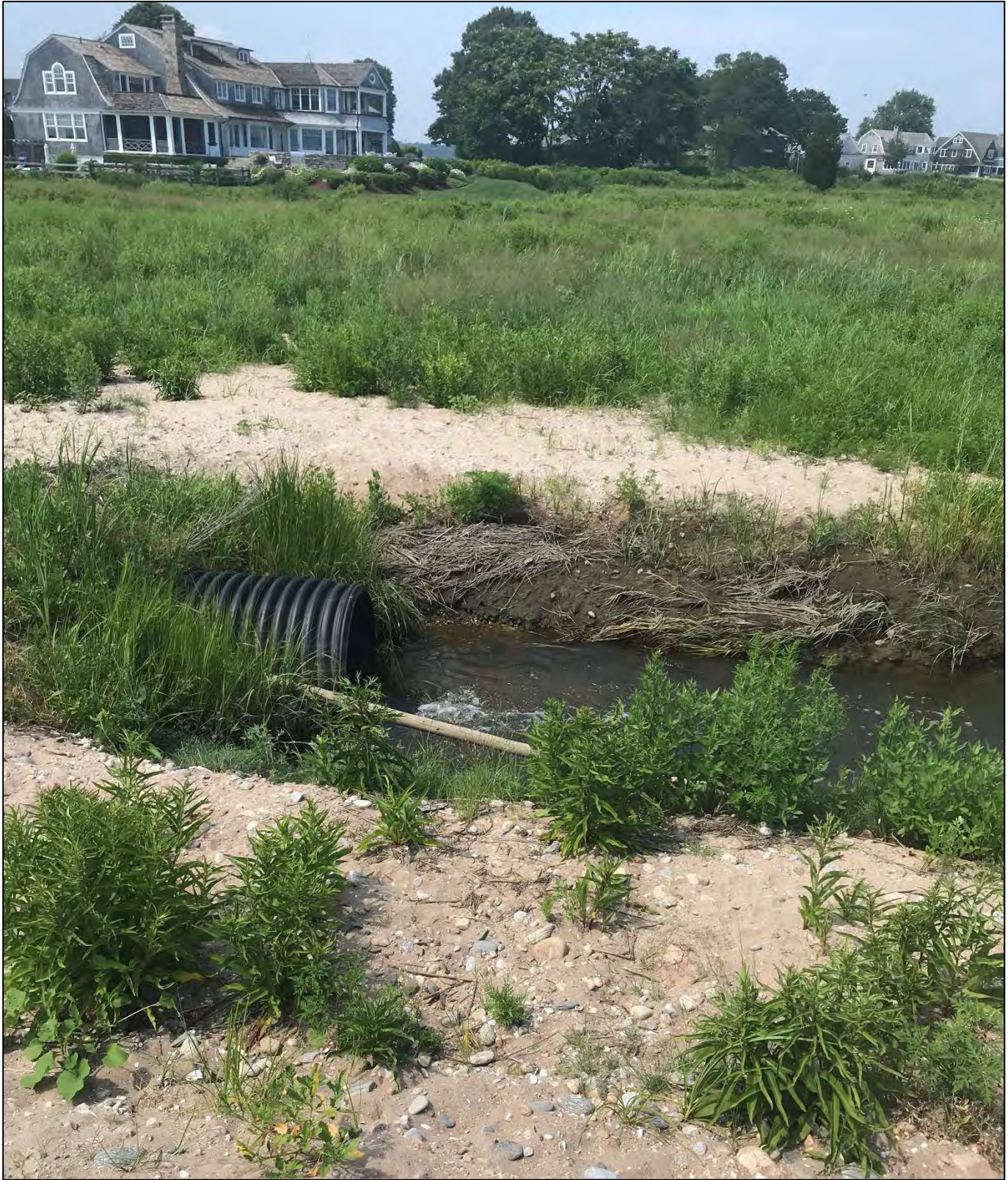
Figure 15 2019 Winter Storm Emergency Response Project: Corrugated pipe (eastern end of the pipe) during ebb flow conditions
