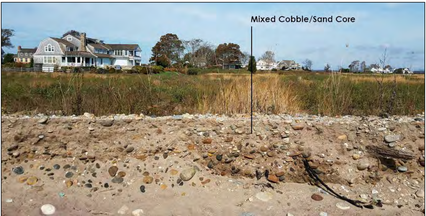
Figure 9 Cobble/Sand composition of existing Hepburn Dune shown after storm-induced erosion (looking north, pre-2019 dune breach)
