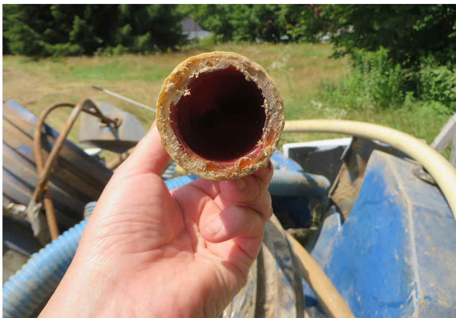
Figure 2. Total Containment Enviroflex pipe unearthed during piping removal. NHDES had required such piping to be removed from UST systems due to ethanol compatibility concerns.
