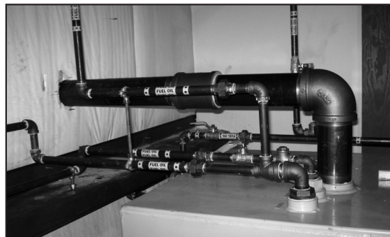
Typical supply and return piping from a tank.
