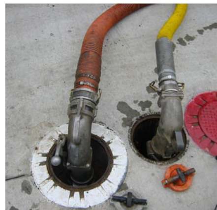
Figure 1. Two-point Stage I vapor recovery requires two separate openings into the tank. In this photo, the hose on the left is for product, the one on the right is for vapors.
